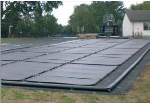
Open space installation
